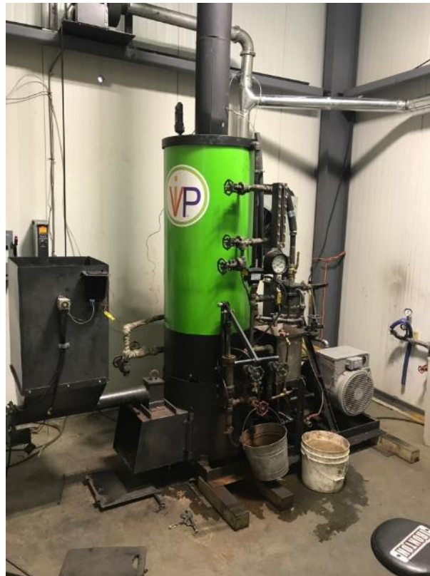
Figure 9: VIP 10-40 Unit in the USA. Note the steam boiler body in green and feedstock hopper on left in black
